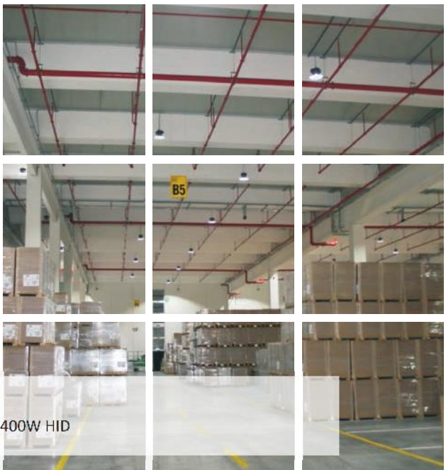
Location: Warehouse, Germany Item: Lumedgo 150W LED high bay light / LMHB-150A / retrofit 400W HID
